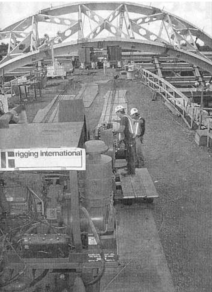
Photo/BRENT BLANCHARD, Rigging International With Rigging International , based in Alameda, Calif., begin lifting Friday on the south abutment of the light-rail bridge over the creek between Delanco and Riverside.
